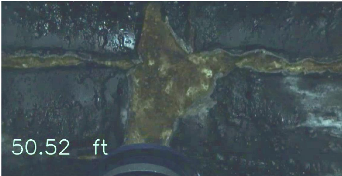
Figure 5. CCTV image of the coal-tar epoxy lining peeling away from the shotcrete below. This image shows the crown of the pipe between the 10 o'clock and 2 o'clock positions.
